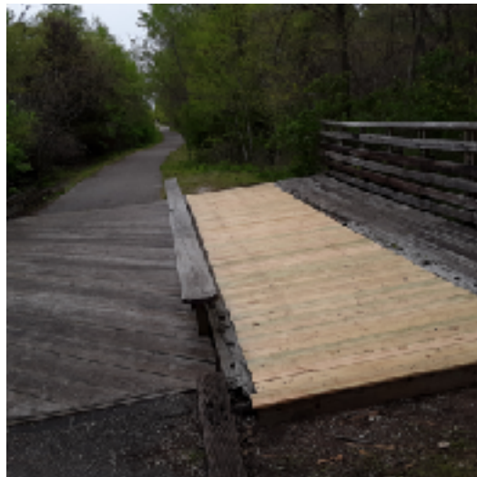
Facing west —bridge rehabilitation is complete before dusk. Primary deck is on the left and north deck on the right. The two are separated by a bench. (Image by Bruce Fingerhut)
