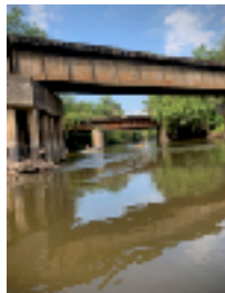
Looking downstream: Former C&O Bridge in The foreground and Former Pennsylvania Bridge in the background.
