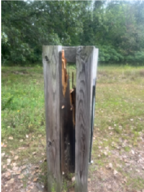
Northern structure of west gate with decayed remnants of horizontal arm (shown in the lifted position). Image by Kathy taken August 8.
