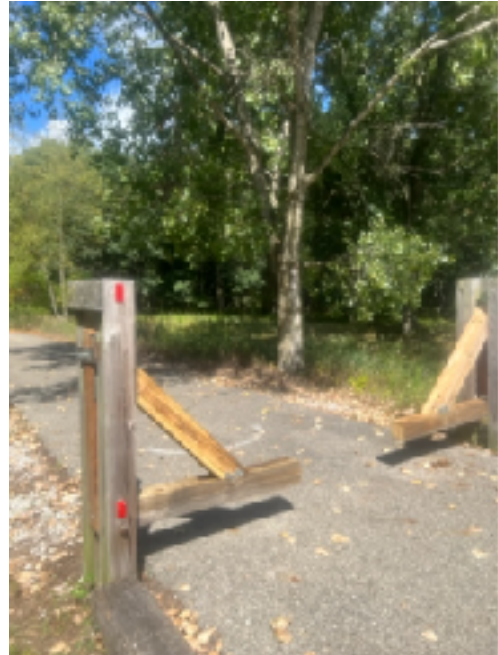
Gate following work by Bruce in 2022 on both arms (shown in the down position). Image by Kathy taken August 20.
