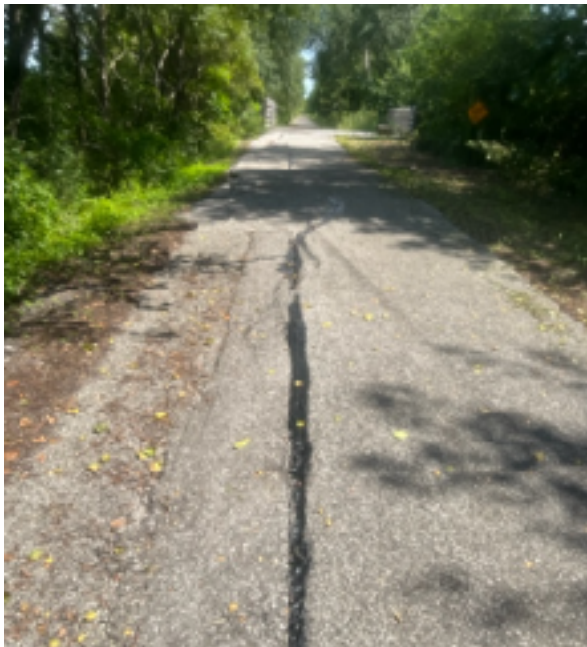
Image of a major asphalt crack filled by Paul Byer using the new rubber applicator. Fell Ditch Bridge is visible in the background.
